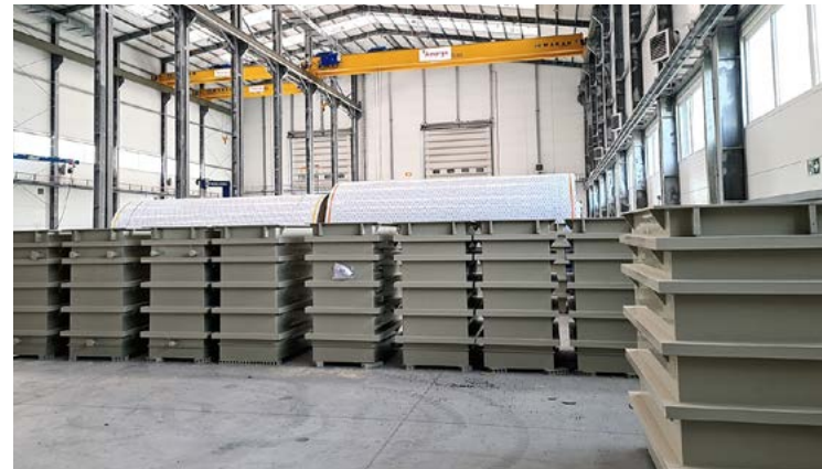
Process tanks (pickling tanks) with equipment and piping for automated production line of metal parts
