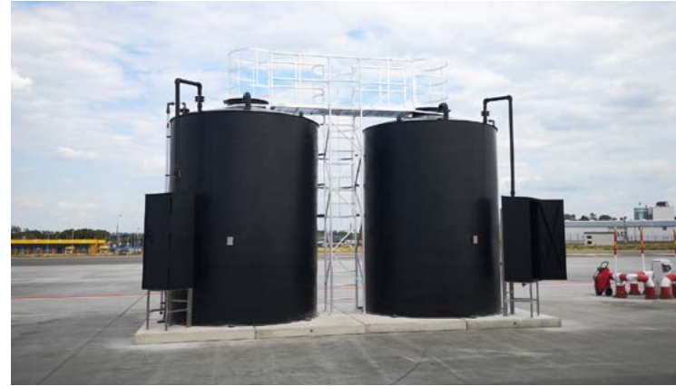
PE100 tanks of 24 m 3 each for storage of Clariant fluid
