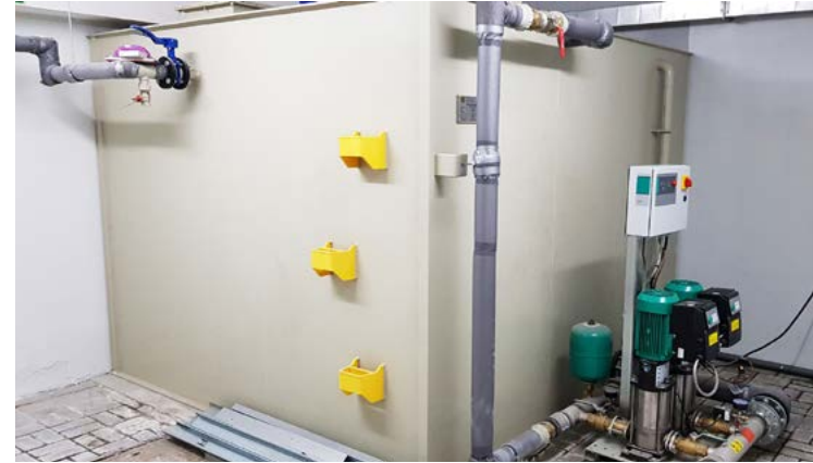
Water reserve tank with a capacity of 10 m 3 for the hospital
