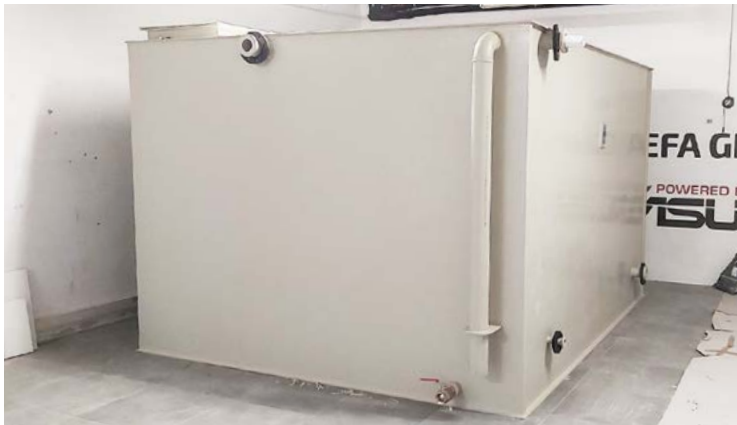
Fire tank of 18 m 3 for the office building
