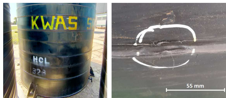
Figure 6. Chemical storage tank for concentrated hydrochloric acid and a crack found in weld of PE layers.
